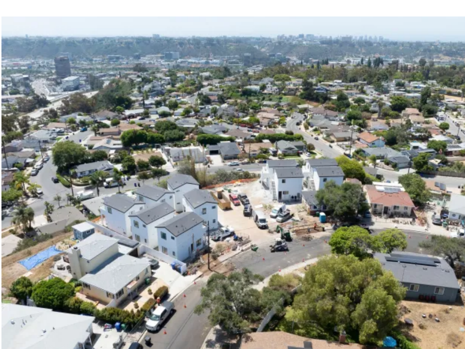
An ADU construction site in Linda Vista on Wednesday, July 9, 2025, in San Diego. (Nelvin C. Cepeda / The San Diego Union-Tribune)
