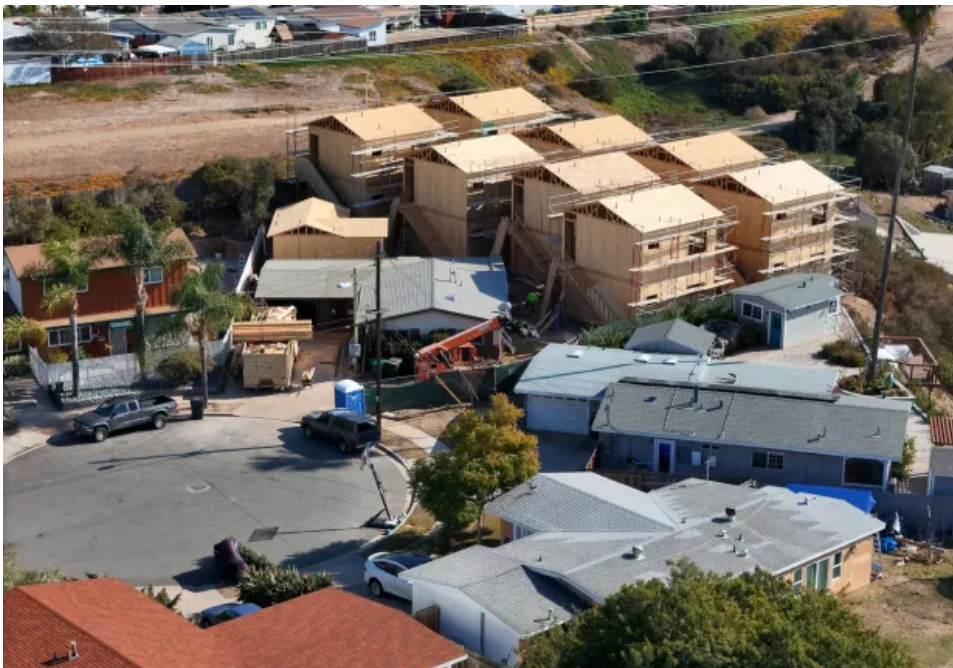
A 17-unit ADU bonus program project being built on Almayo Avenue in Clairemont on Wednesday, Jan. 29, 2025. The lot originally housed a 1,018-square-foot single-family home. (K.C. Alfred / The San Diego Union-Tribune)
